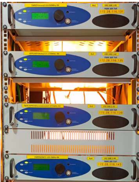
CNS facilities | VHF transmitter & receiver
